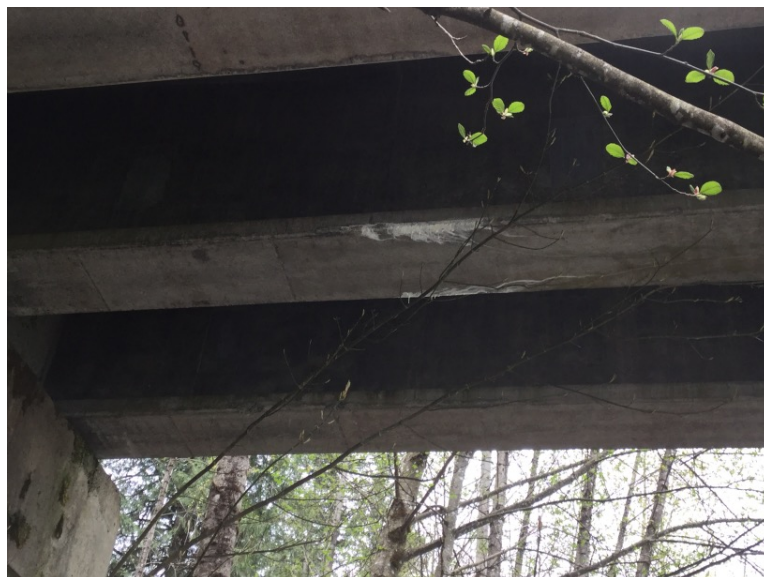
Effluence on center girder near left pier
